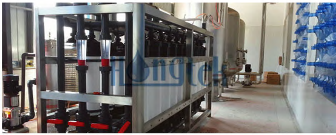
Mineral water ultrafiltration equipment 40m 3 /h
